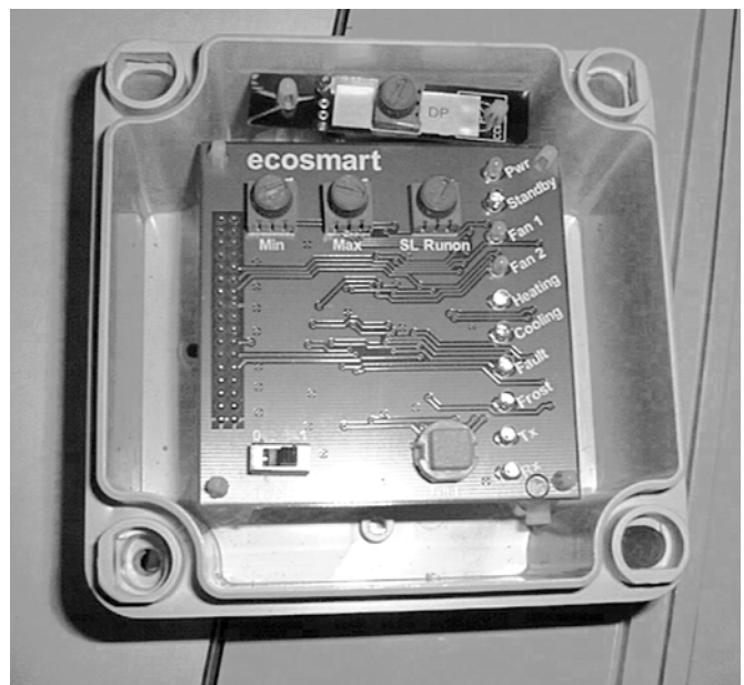
Figure 5. Fan side commissioning box.
